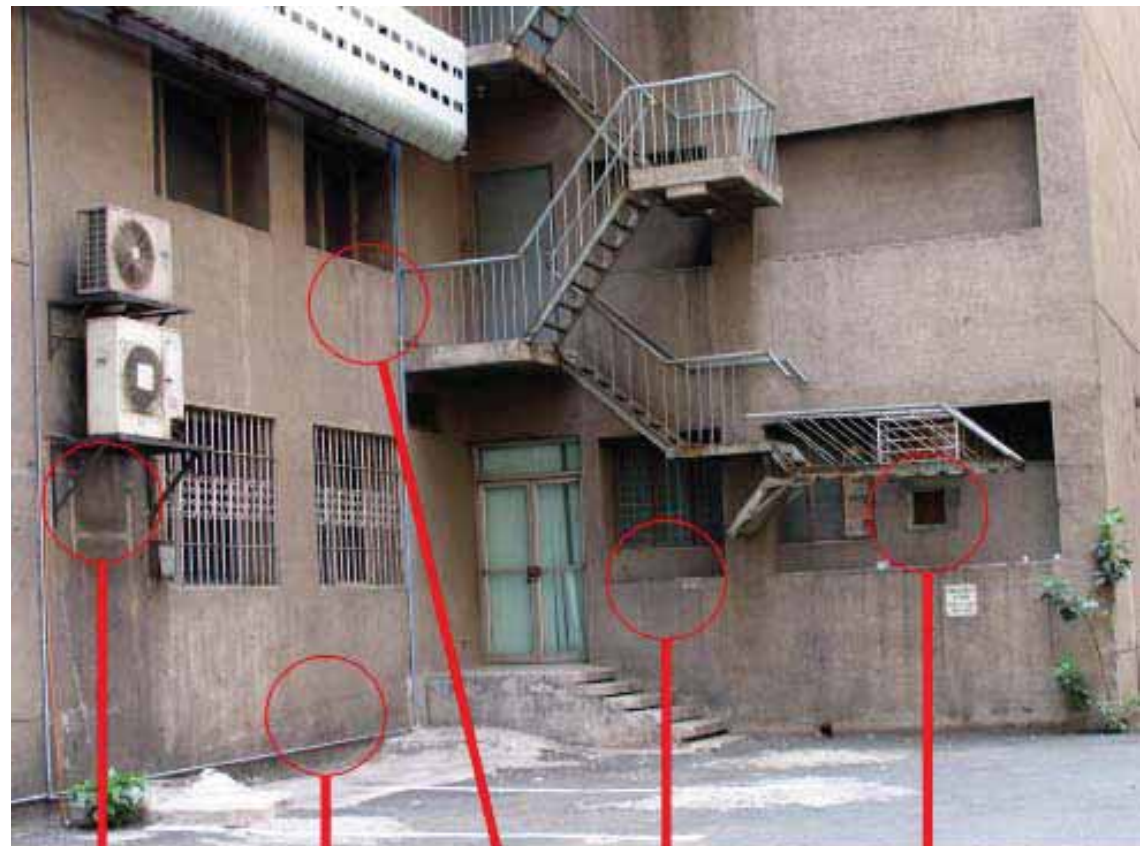
Dirt and water from A/C system
